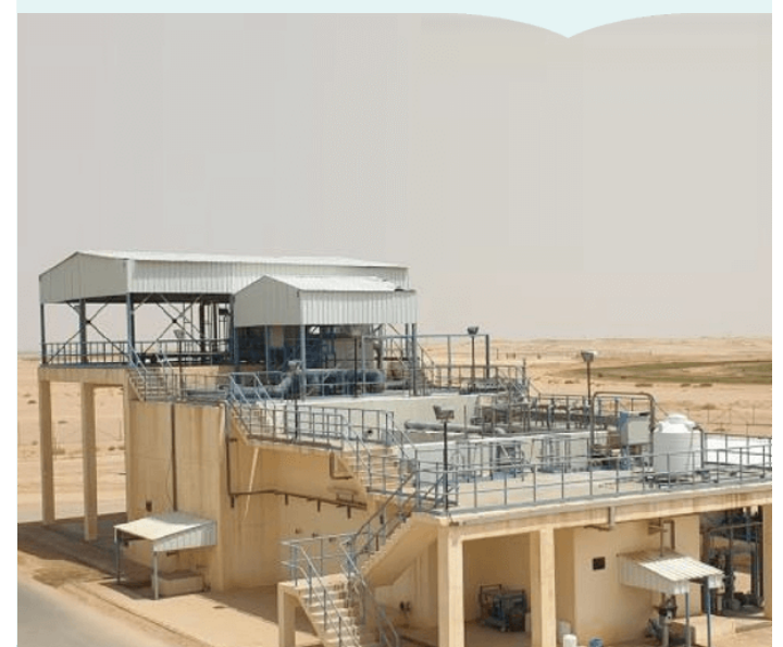
Effluent Treatment Plant (ETP) - Al Kharj
